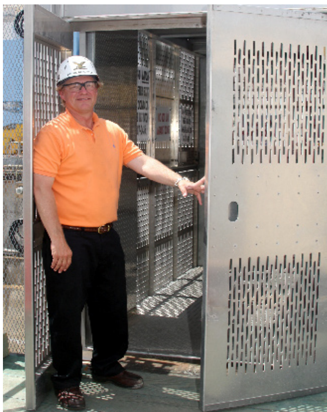
FOUR TO THE FLOOR—USS TENNESSEE (SSBN 734) Project Superintendent Dennis Bevington demonstrates the new Dry Dock 4 elevator that carries personnel and equipment to and from the TENNESSEE project. The elevator is permitted to carry up to 6,000 lbs. (or 30 people).
